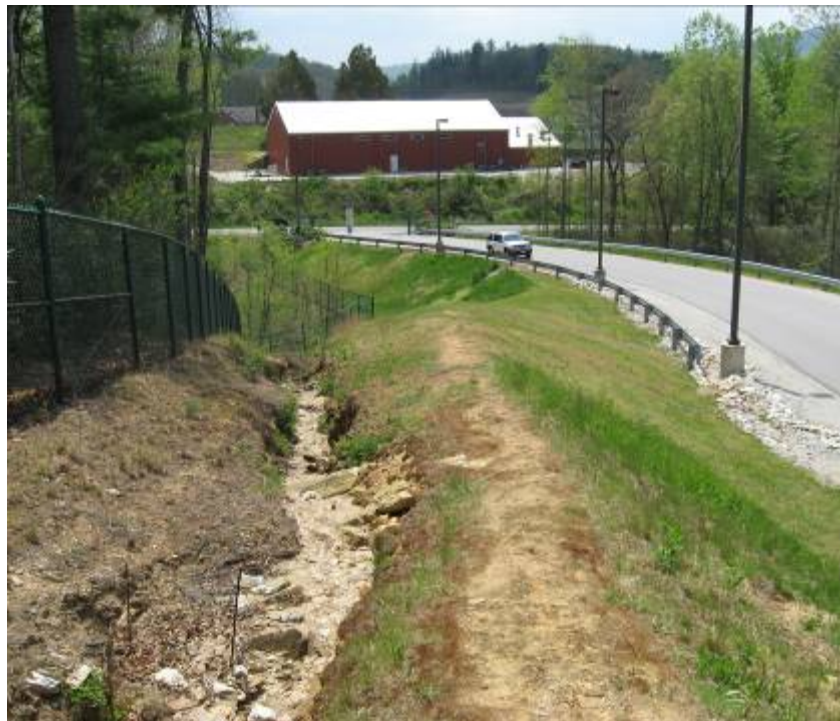
Photograph 2 – Erosion from stormwater runoff from Greenlee School.
