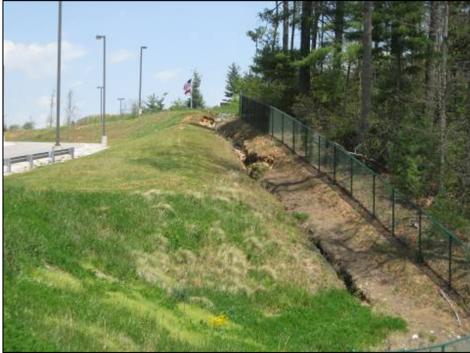
Photograph 1 – Erosion and gully from stormwater pond in front of Greenlee School.
