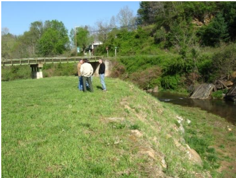
Photograph 2 – Representative view showing limited access to Cane Creek, poor riparian vegetation, and over-steepened bank.
